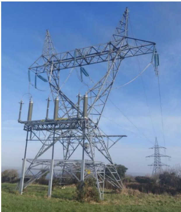
Figure 5.11: Line Cable Interface Mast (LCIM)
